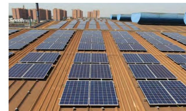
PV power generation system
